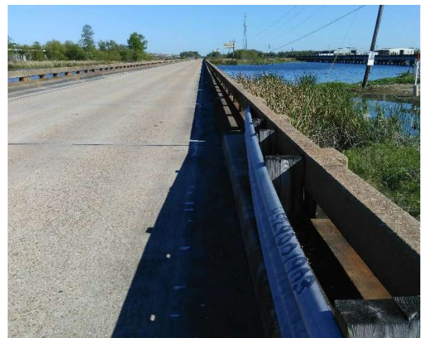
Photograph 3. Old U.S. Highway 51 bridge over North Pass Manchac, facing north. The bridge has two narrow traffic lanes and no shoulders. Currently, Pedestrians or bicyclists must share the road.
